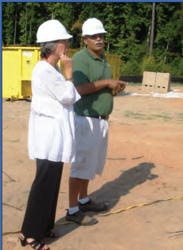
Aug. 22, 2011—Above, TxAire project participant Anwar Khalifa (right) leads EO Libby Simmons on a tour of the building site on the UT Tyler campus. The research project demonstrates different energy saving building techniques.
